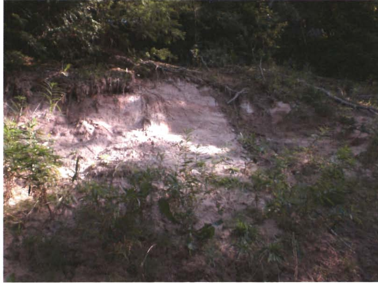
Figure 37: Erosion Site Two
