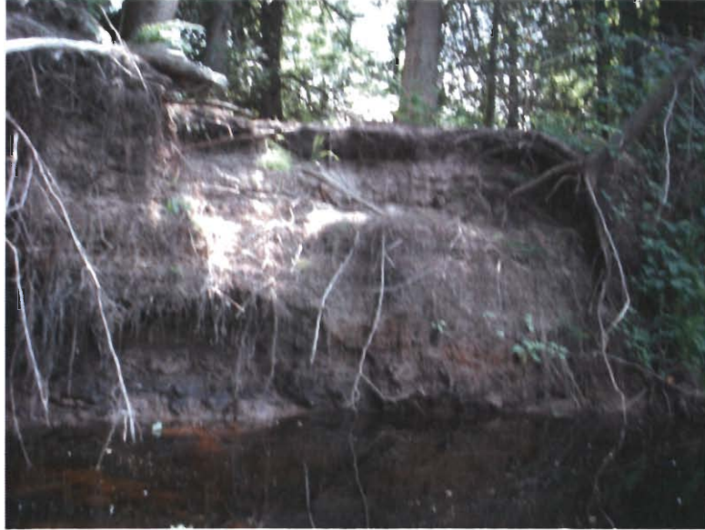
Figure 49: Erosion Site Fourteen
