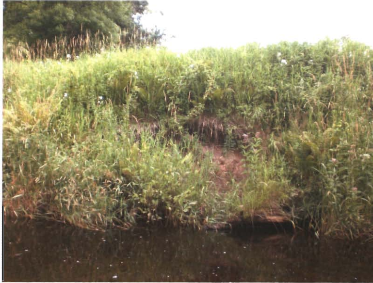
Figure 46: Erosion Site Eleven
