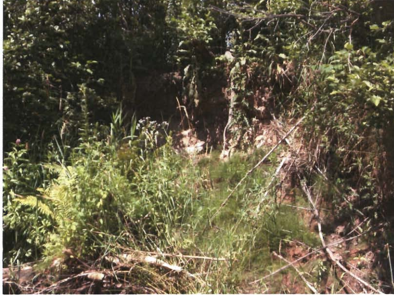
Figure 44: Erosion Site Nine
