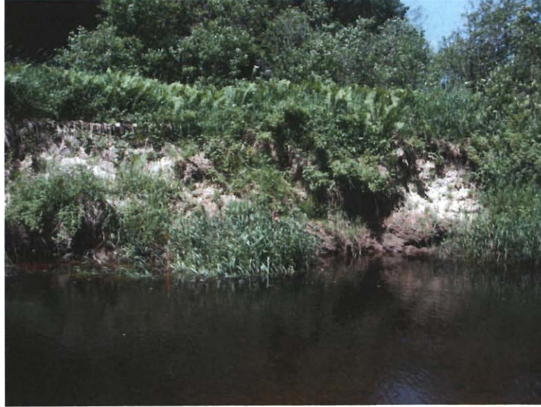
Figure 51: Erosion Site Seventeen
